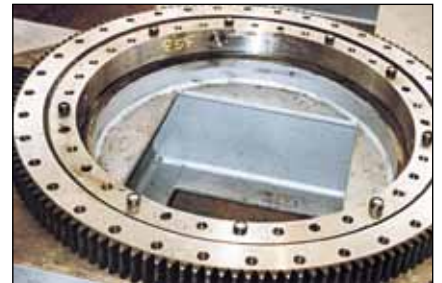
WEICON WR - Underfilling of a live ring in a deck crane installation
